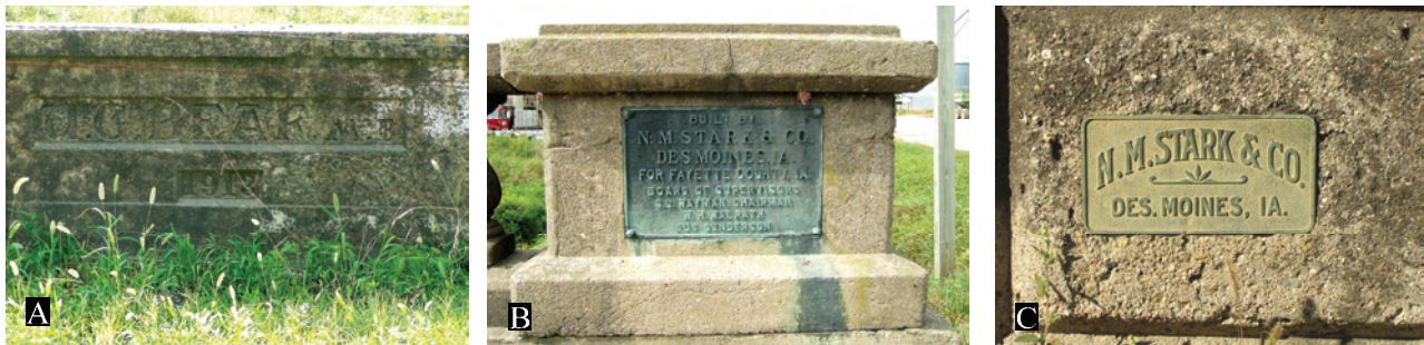
Figure 57. A. The signature 1912 concrete and steel bridge, with impressed “A.G. BEAR, M.B.”, Centerville vicinity, Appanoose County. B. Bronze Stark plaque, West Union, Fayette County. C. The ca. 1913 H. M. Stark & Company bronze bridge plaque in Gifford, Hardin County. 2003 survey photos.
