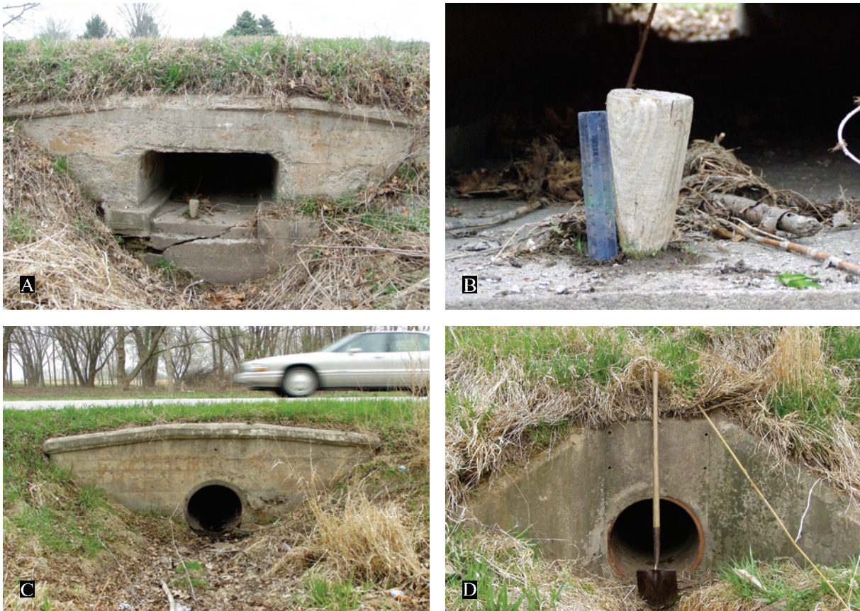
Figure 114. A. View of ca. 1913, cast in place, concrete culvert with low parapet and imbedded, turned-out, wooden wagon wheel hub used as survey point, North Liberty, Johnson County. Note shouldered and stepped base of outlet with chamfered top corners. Cracking and spalling is due to water running under culvert causing cavitation and resultant cracking. B. Detail of axle hub in culvert (6" ruler). C. View of 1913 ceramic tile pipe culvert along Red Ball segment between Iowa River and Shueyville now on old U.S. 218. D. Detail of small, ca. 1930, cast in place concrete, wing type headwall outlet with ceramic tile pipe culvert on old 218 south of Iowa City. 2003 survey photos.
