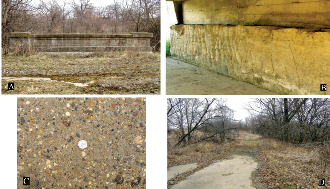
Figure 94. A. View of cut-off segment showing bridge/culvert. B. Detail of bridge footings showing spade marks. C. Detail of concrete pavement. D. View of obliterated segment through field. 2003 survey photos.
