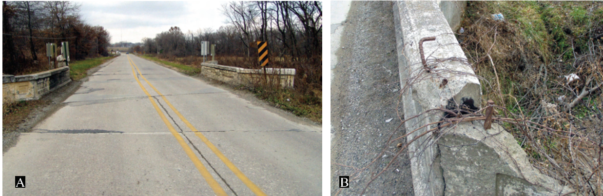
Figure 97. A. View of ca. 1916 culvert on old Iowa 8/U.S. 34 in southwest Ottumwa, Wapello County. B. Detail of concrete showing both twisted and rectangular rebar. 2003 survey photos.
