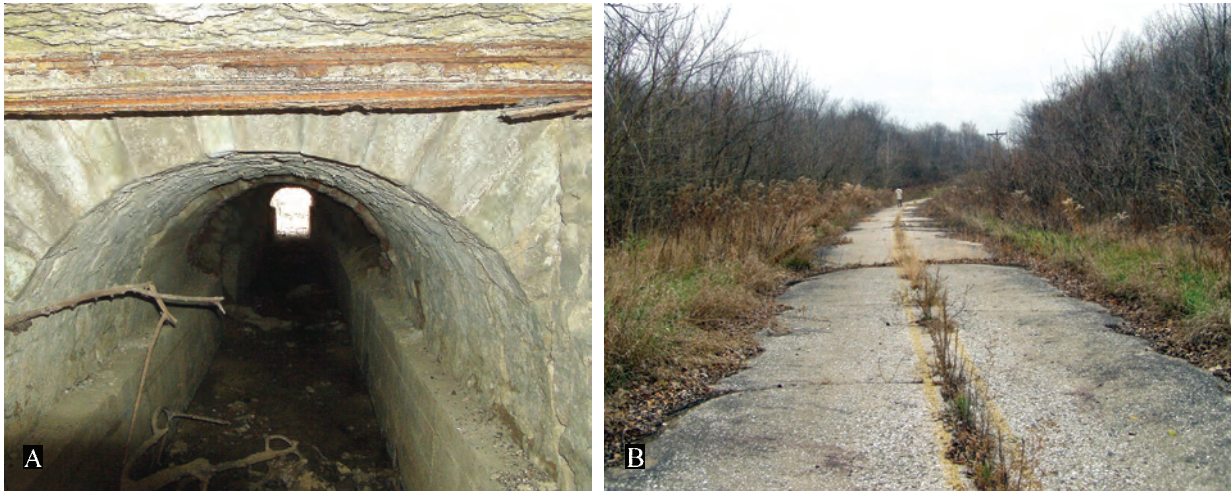
Figure 96. A. Detail of interior of cut limestone culvert adapted from 1869 railroad spur (Section G; Segment 1) showing stonework, concrete and brick lining, and iron support bars. B. View of cut-off and abandoned segment (Section G; Segment 2) looking southwest. 2004 survey photos.
