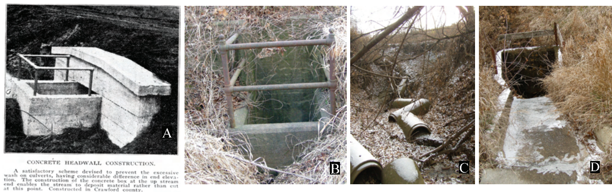
Figure 54. A. Drop culvert concrete headwall construction of Crawford County culvert (ISHC 1915c:78). Note parapet top. B. Drop culvert (ca. 1920) with raised top rails made of iron boiler pipe to prevent debris accumulation and as cattle guard near Albia, Jefferson County. C. Eroded and collapsed large tile pipe spillway culvert outlet near Albia. D. Concrete gutter from curb drain to drop culvert (top of C) with wooden rail surround, old U.S. 34, Albia vicinity, Monroe County (B–D 2003 survey photos).
