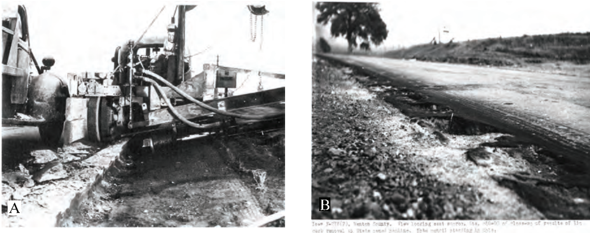
Figure 63. A. Curb removal machine ca. 1950 (Iowa DOT 1997:41). Note size of spalls removed. B. Benton County highway showing scars of curb removal in 1949 (Iowa DOT Library-Photos).
