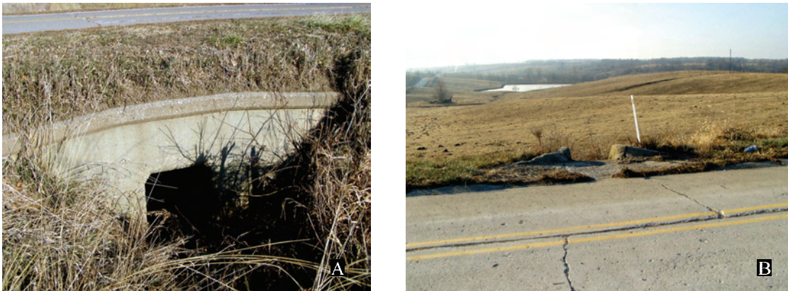
Figure 101. A. View of early parapet topped culvert on old Iowa 8/U.S. 34 atop ridge. B. View of ridge top route of old Iowa 8/U.S. 34 with integral lip-curb drain (now county road H35). 2003 survey photos.
