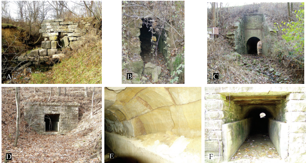
Figure 41. A. Jockey Hollow stone bridge. B. Jockey Hollow stone culvert. C. Stone and concrete culvert with associated stone-lined drainage. D.–F. Stone culvert and details of same, Ottumwa vicinity, Wapello County (2003 survey photos).
