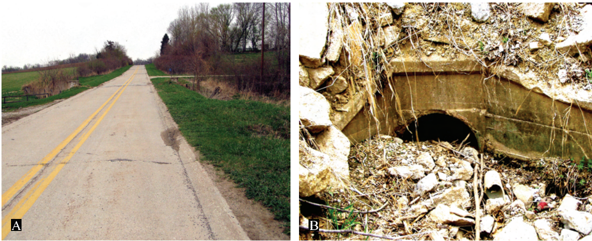
Figure 115. A. View of in-use cut-off segment from old U.S. 218 (South Curtis Bridge Road) north to the Iowa River showing original 1920s cross-section, pavement with integral lip-curbs, and structures. B. View of original parapet top wing wall culvert south of Shueyville, Johnson County (North Curtis Bridge Road) that pre-dates concrete paving. Note color. Culvert is covered with debris from curb removal.
