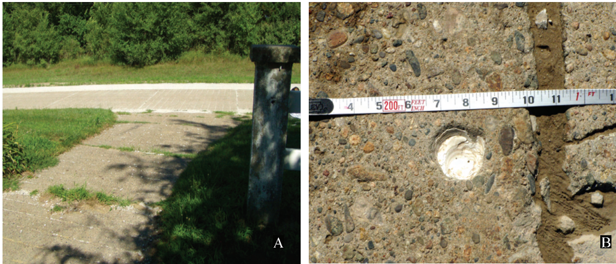
Figure 70. A. View of Eddyville Cemetery's concrete pavement (2003 survey photo) with scored 14 ft long sections. B. Detail of Eddyville cemetery pavement. Note shell in aggregate. 2003 survey photos.
