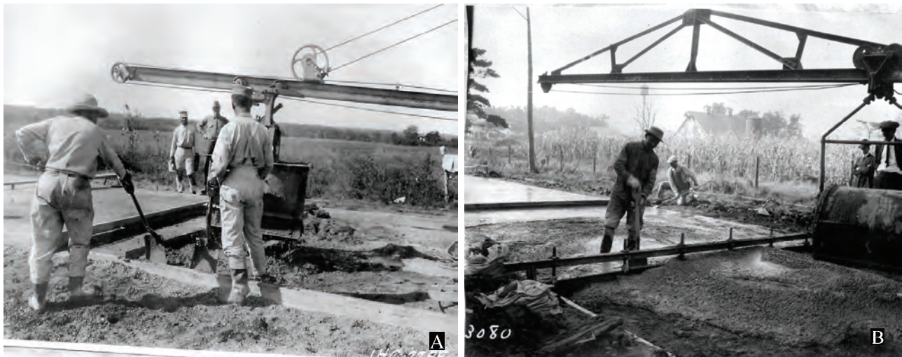
Figure 48. A. Concrete paving of Fredonia to Columbus Junction road with forms in place (ISHC 1914c). B. Pour in progress (ISHC 1914d) (Photos #2255 and #3080, Iowa DOT Library).
