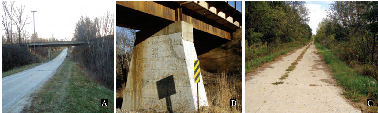
Figure 100. A. View of dated 1927 railroad trestle over old U.S. 34. B. Detail of trestle. Note newer concrete top. C. View of cut-off segment of old U.S. 34 dead ending at Cedar Creek. 2003 survey photos.
