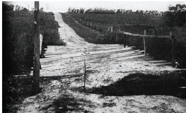
Figure 33. Woodward plank and pole bridge declared “Death Trap” (Road-Maker 1916m:7).
