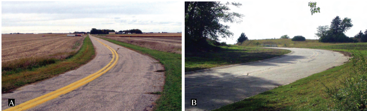
Figure 47. A. Mooned-Out curve on old U.S. 18 west of Algona, Kossuth County. B. Supra-elevated curve on integral lip-curbed section of old U.S. 20 east of Sioux City, Woodbury County. 2003 survey photos.
