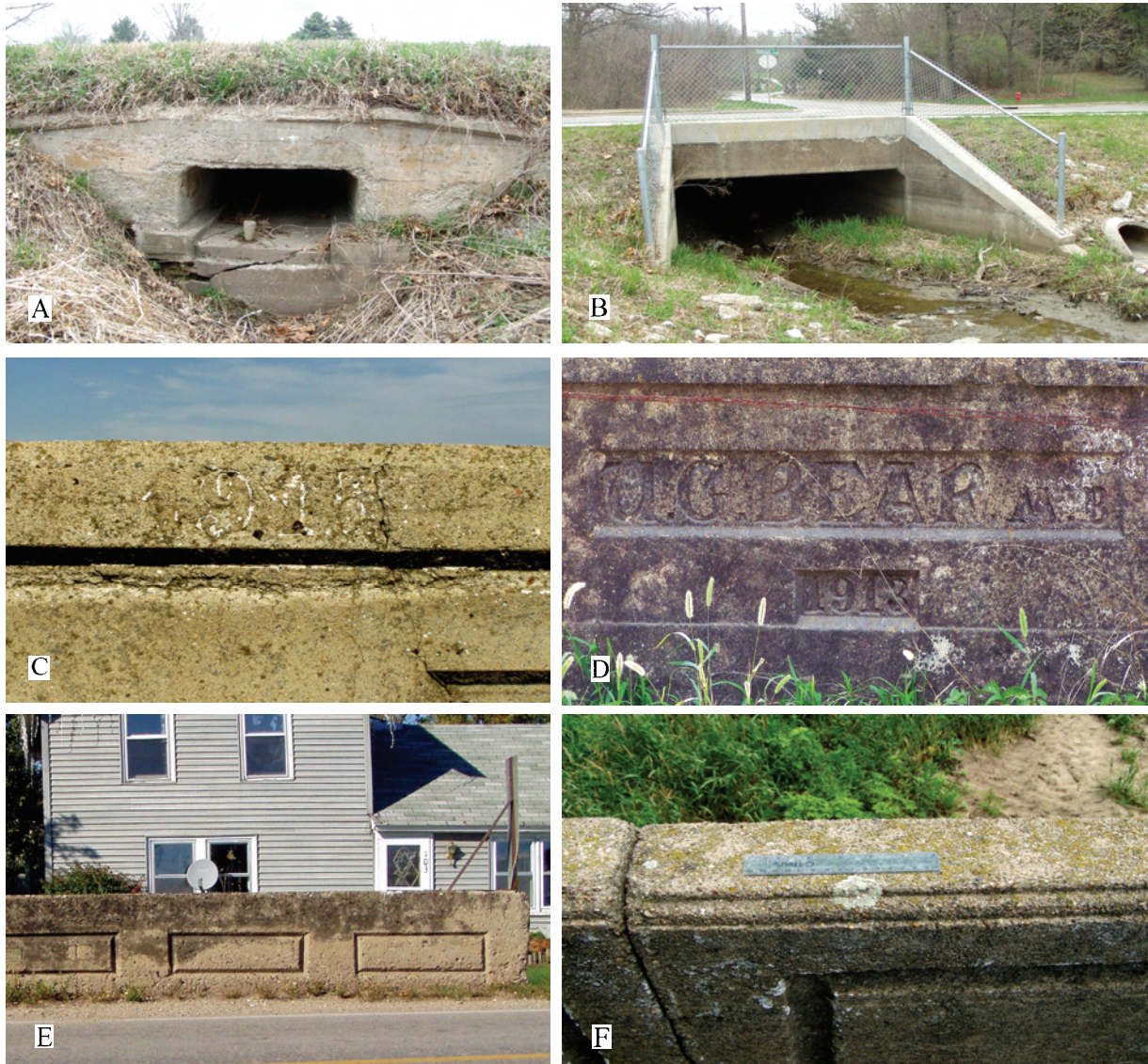
Figure 82. Pre-1920 concrete color variation examples. A. Circa 1913 Red Ball culvert, North Liberty, Johnson County. Note wooden wagon axel hub used as survey point. B. New concrete over old from the 1911 Red Ball culvert on Dubuque Street, Iowa City, Johnson County. C. A 1915 culvert just west of Correctionville, Woodbury County. D. A. G. Bear's 1913 bridge rail, Centerville, Appanoose County. E. Circa 1913 bridge handrail, Gifford, Hardin County by Stark Co., nonextant 2008. F. Detail of ca. 1913 Marsh arch bridge rail and panel, Dunkerton, Black Hawk County (2003 survey photos and 6" ruler).
