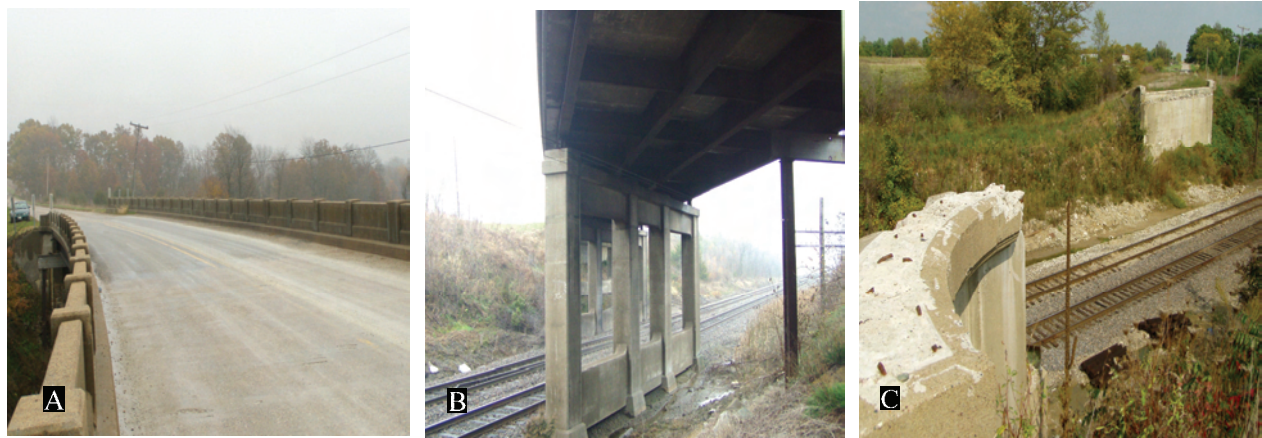
Figure 91. A. View of the now nonextant, curved, ca. 1930, Art Moderne-styled concrete railroad overpass. B. View of deteriorated bridge supports. 2003 survey photos. C. View of obliterated bridge's headwalls (2005 photo).
