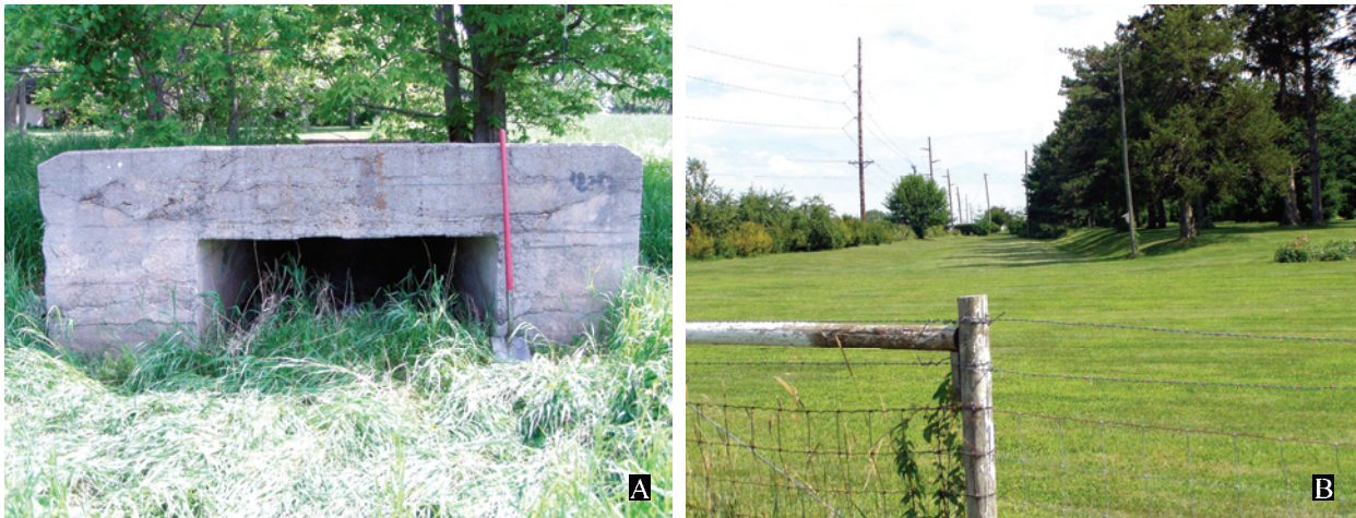
Figure 112. A. Hog crossing culvert (1915) abandoned next to farmstead. Note lack of siderail. Approaches are gone. B. View of 1915 road bed cut along edge of farmstead. 2003 survey photos.
